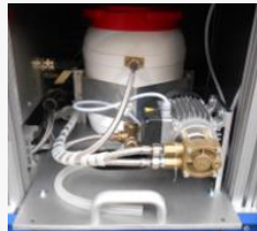
Water tank and pump
